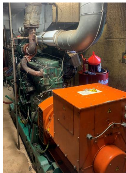
Figure 1. Dual fuel engine at Hedeland, Denmark, using landfill gas as main fuel and diesel as pilot fuel.
